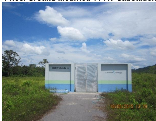
Gambar 1.10 1 nos. Ground Mounted 11 KV Substation
